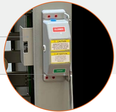
DOOR INTERLOCK TO PREVENT OPENING OF EXTERIOR DOOR WITH SWITCH IN ON POSITION
