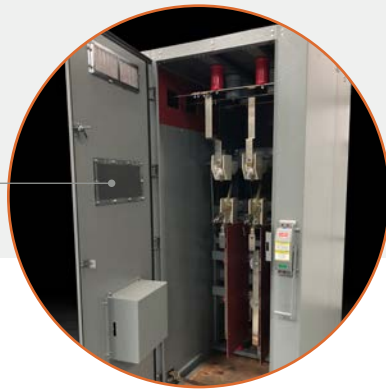
VIEWING WINDOW TO VIEW SWITCH POSITION FOR SAFETY
