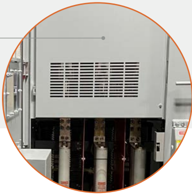
GROUNDING BARRIER FOR PROTECTION FROM LIVE VOLTAGES
